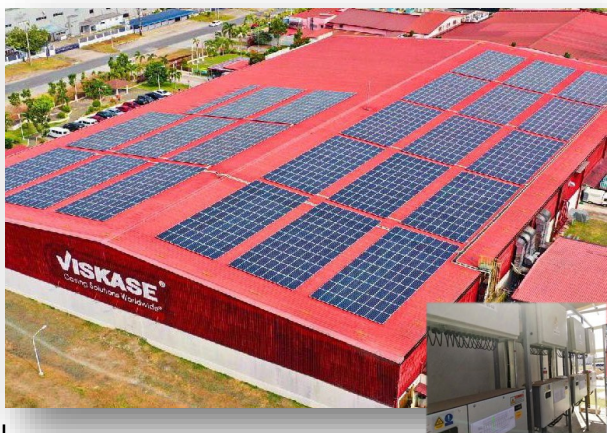
Philippines Capacity: 604.5 kWp Inverter Model: SUN2000-42KTL
