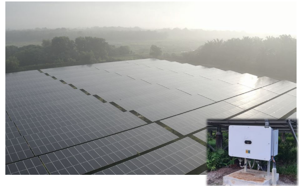
Kamunting, Perak Ground-mounted Smart PV Plant Capacity: 30 MW Inverter Model: SUN2000-185KTL-H1
