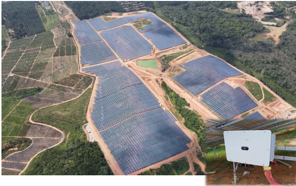
Pasir Gudang, Johor Ground-mounted Smart PV Plant Capacity: 25 MW Inverter Model: SUN2000-185KTL-H1
