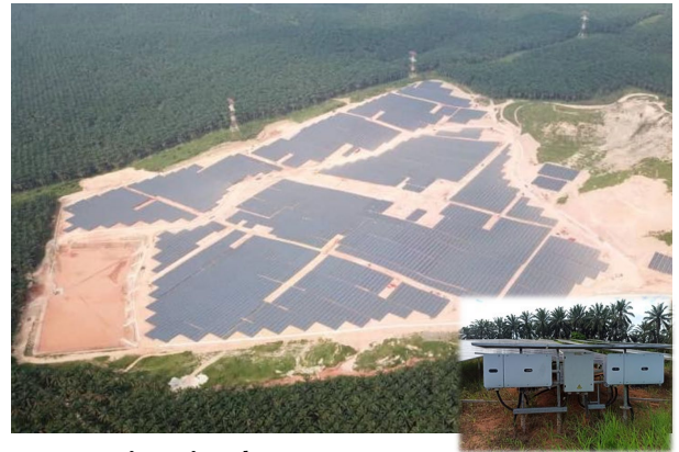
Kota Tinggi, Johor Ground-mounted Smart PV Plant Capacity: 29 MW Inverter Model: SUN2000-90KTL-H1
