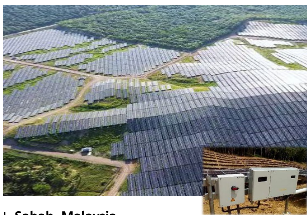
Sabah, Malaysia Mountain-mounted Smart PV Plant Capacity: 49 MW Inverter Model: SUN2000-42KTL
