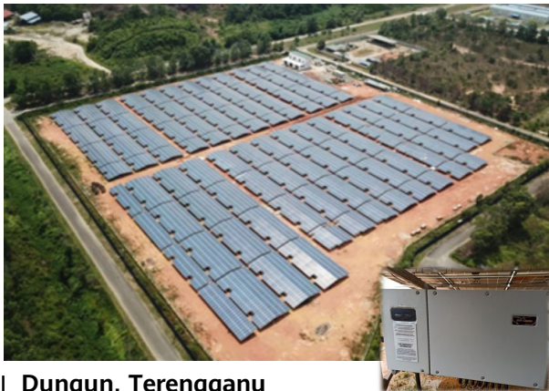
Dungun, Terengganu Ground-mounted Smart PV Plant Capacity: 43.5MW Inverter Model: SUN2000-42KTL
