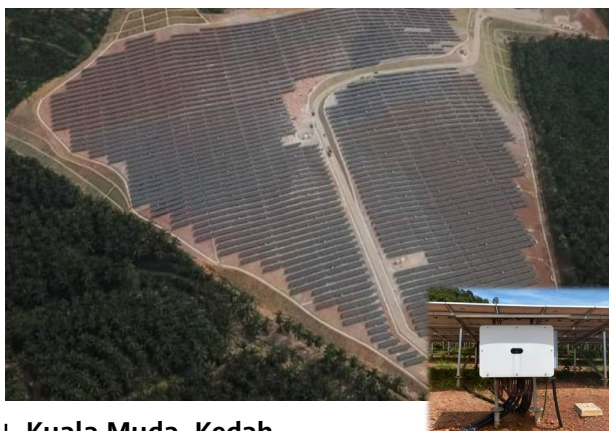
Kuala Muda, Kedah Ground-mounted Smart PV Plant Capacity: 30 MW Inverter Model: SUN2000-185KTL
