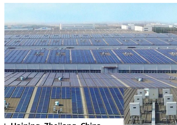
Haining, Zhejiang, China Largest Rooftop-mounted PV Plant Worldwide Capacity: 300 MW Inverter Model: SUN2000-28KTL, 36KTL, 50KTL
