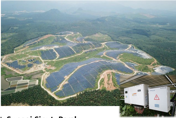
Sungai Siput, Perak Ground-mounted Smart PV Plant Capacity: 49 MW Inverter Model: SUN2000-42KTL
