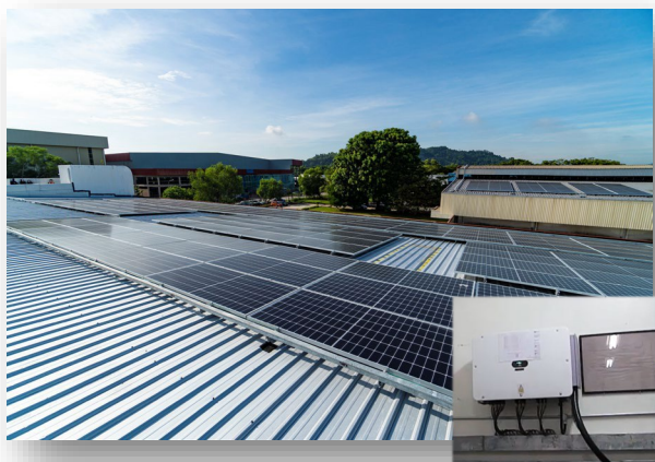
Malaysia Capacity: 0.6 MW Inverter Model: SUN2000-36KTL
