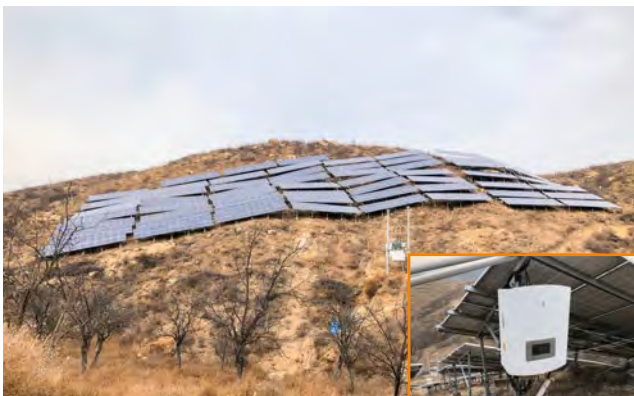
Hebei Baoding Fuping poverty alleviation PV Plant 6.6MW
