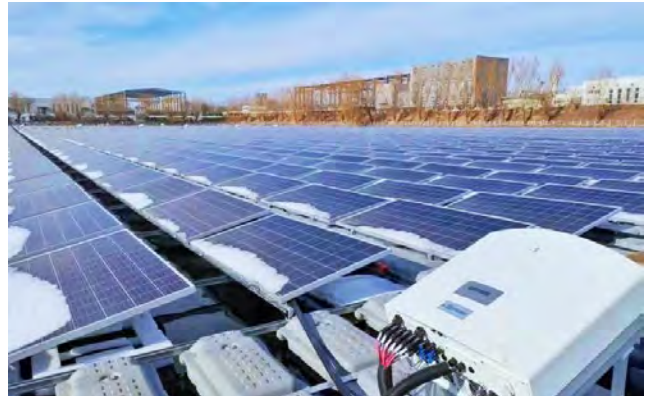
Beijing Shunzhen Green Harbor's Plant 5.5MW
