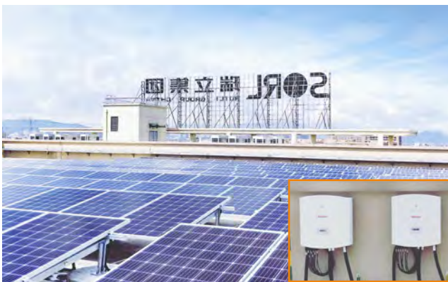
Zhejiang SORJ 3.9MW
