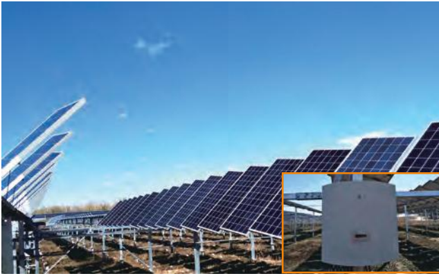
Hebei Zhangbei Agricultural-photovoltaic hybrid PV plant 50MW
