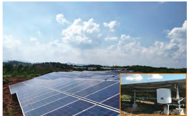
Jiangxi Ganzhou PV Plant 3.5MW
