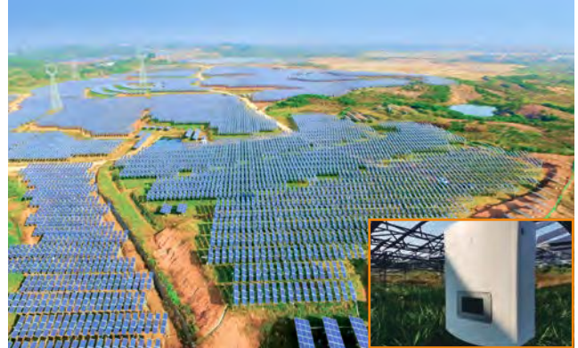
Zhejiang Hangbu Agricultural-photovoltaic hybrid PV plant 30MW
