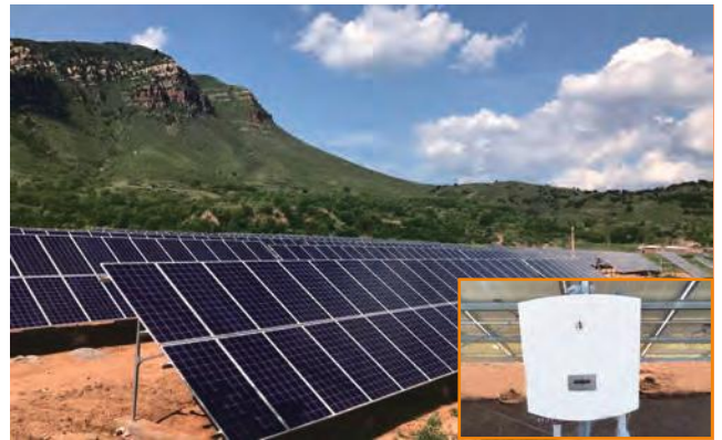
Shanxi Xiyang poverty alleviation PV Plant 7.2MW
