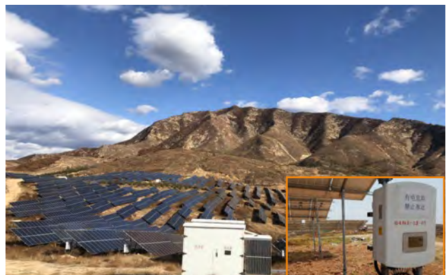
Liaoning Gaizhou Jiuzhai PV plant 20MW
