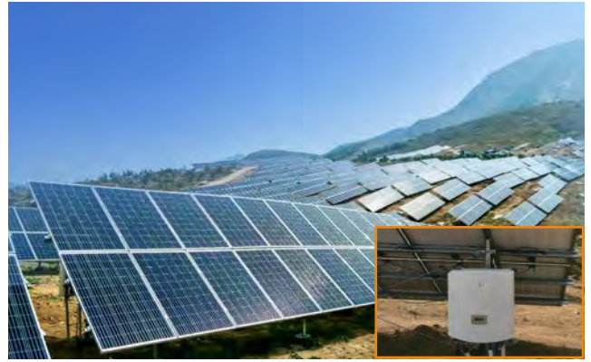
Liaoning Yingkou Jiuzhai PV plant 20MW
