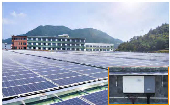
Tyco Electric, Panan Jinhua Zhejiang 1.5MW
