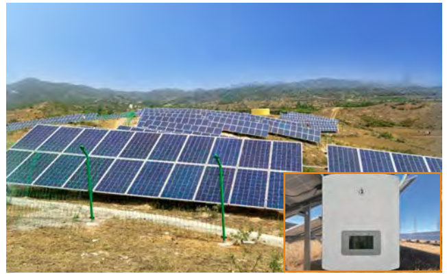
Hebei Qinghuangdao poverty alleviation PV Plant 9.7MW
