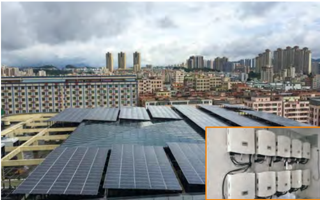
Shenzhen Jiangnan Times Building 600kW
