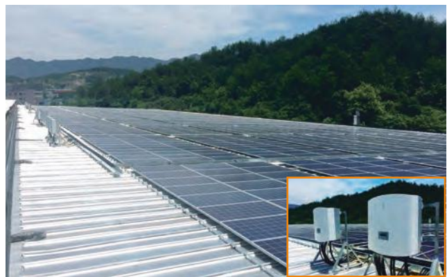
Hainan JiuLongGlass 1.7MW
