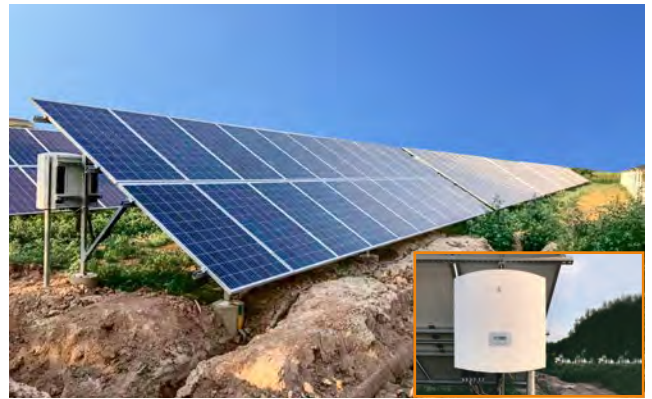
Hebei Qinghuangdao poverty alleviation PV Plant 5MW
