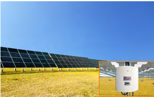
Huaneng Yimin surface mine PV plant 20MW
