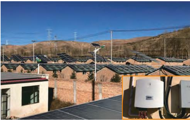
Qinghai HuzhuBanyan poverty alleviation PV Plant 2MW
