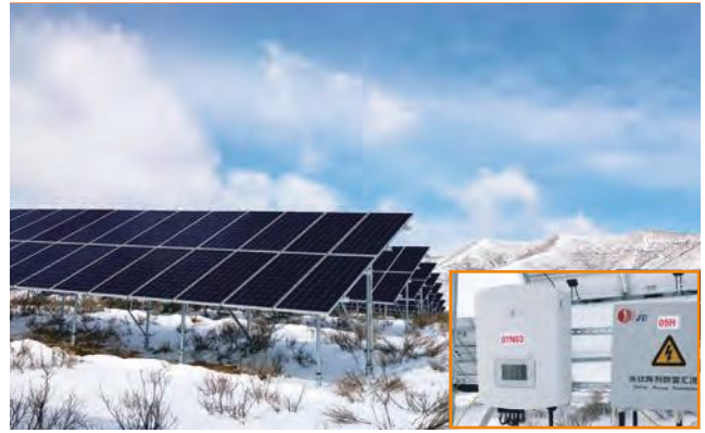
Shanxi Guangling PV plant 1.47MW
