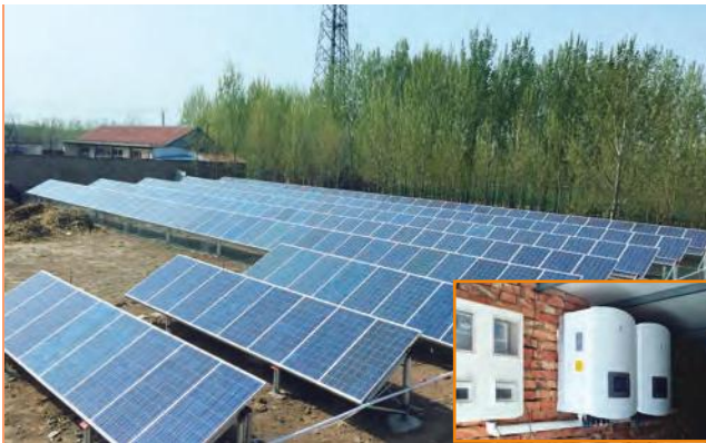
Shandong Leling poverty alleviation PV Plant 50kW
