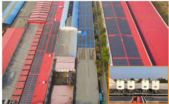
Shandong Weifang Linqupoverty alleviation PV Plant 20MW
