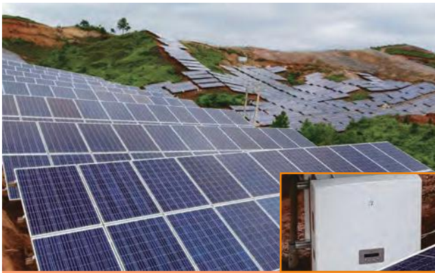
Jiangxi Ganzhou Hengjiang poverty alleviation PV Plant 8.45MW
