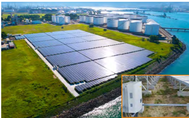
JTC Solar Farm, Singapore 5MW
