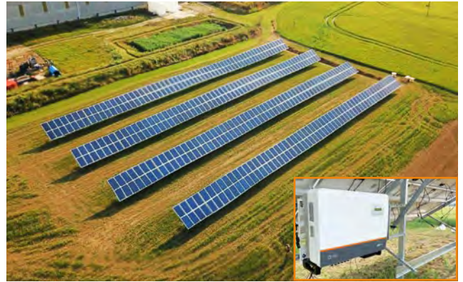
Lincolnshire, UK 140kW
